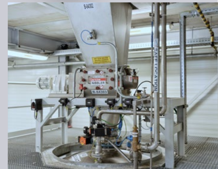
Calibration of raw material upstream of reactor vessel
