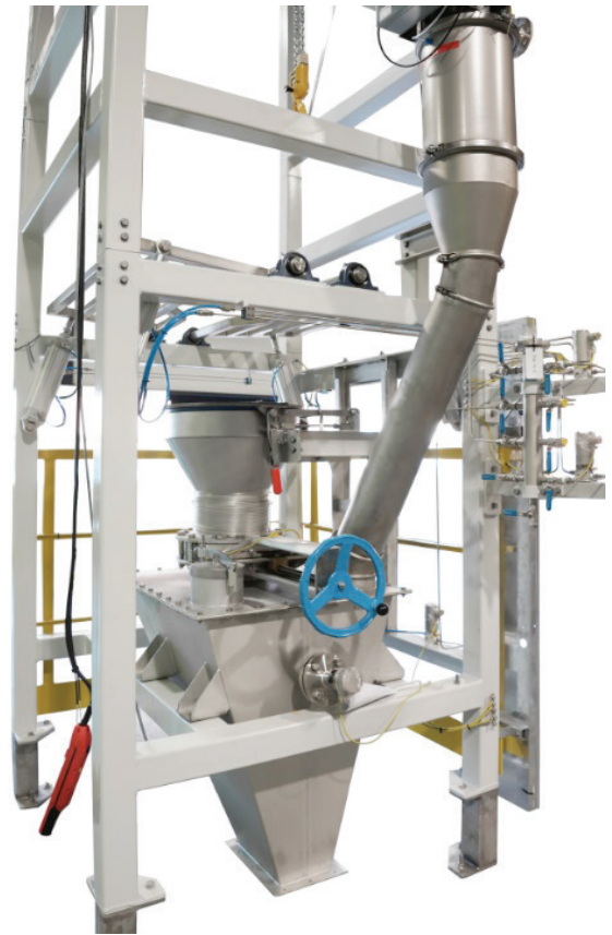
Close up of BBU docking station, hopper and GDU 201.3
