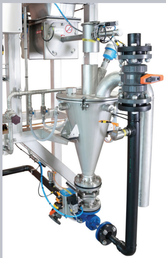
Feeder > vortex vessel attached to a eductor
